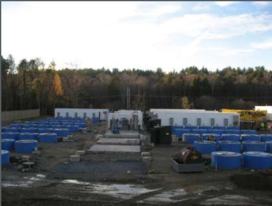
Beacon Power Flywheel Facility, Stephentown, NY
