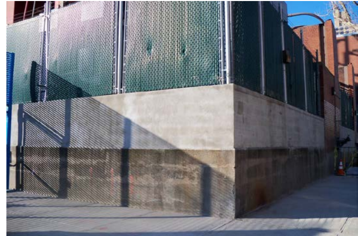
Raised concrete walls protecting critical equipment
